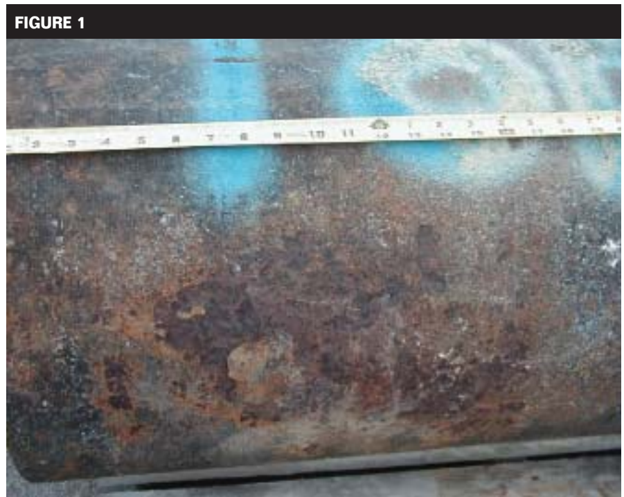
Corrosive attack to 16-in. water main (71% wall max. pit depths).
